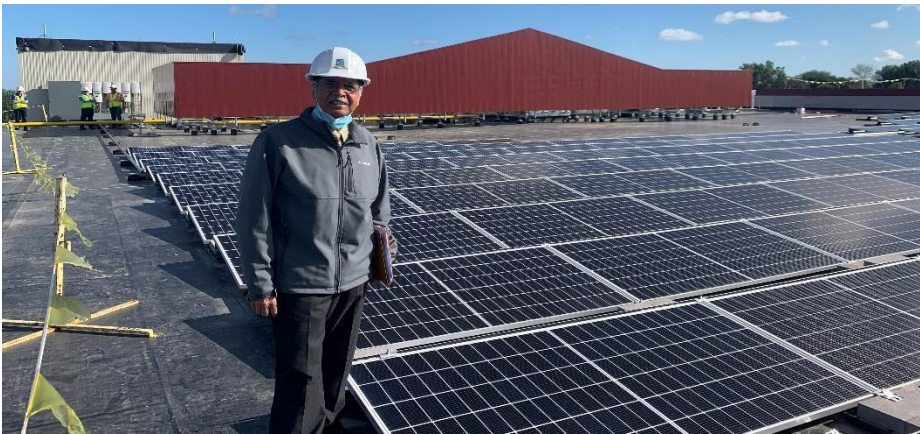
Town of Greece – Greece Central School District – Bus Maintenance Garage Solar Array
