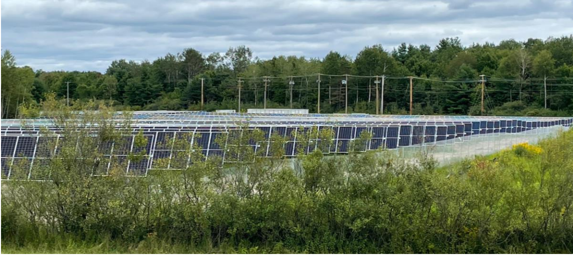
Richland Community Solar Project
